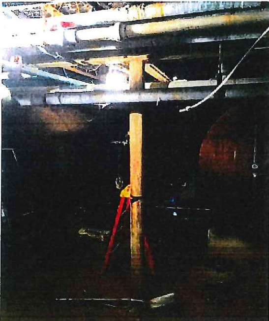
Existing Water System & Tanks
